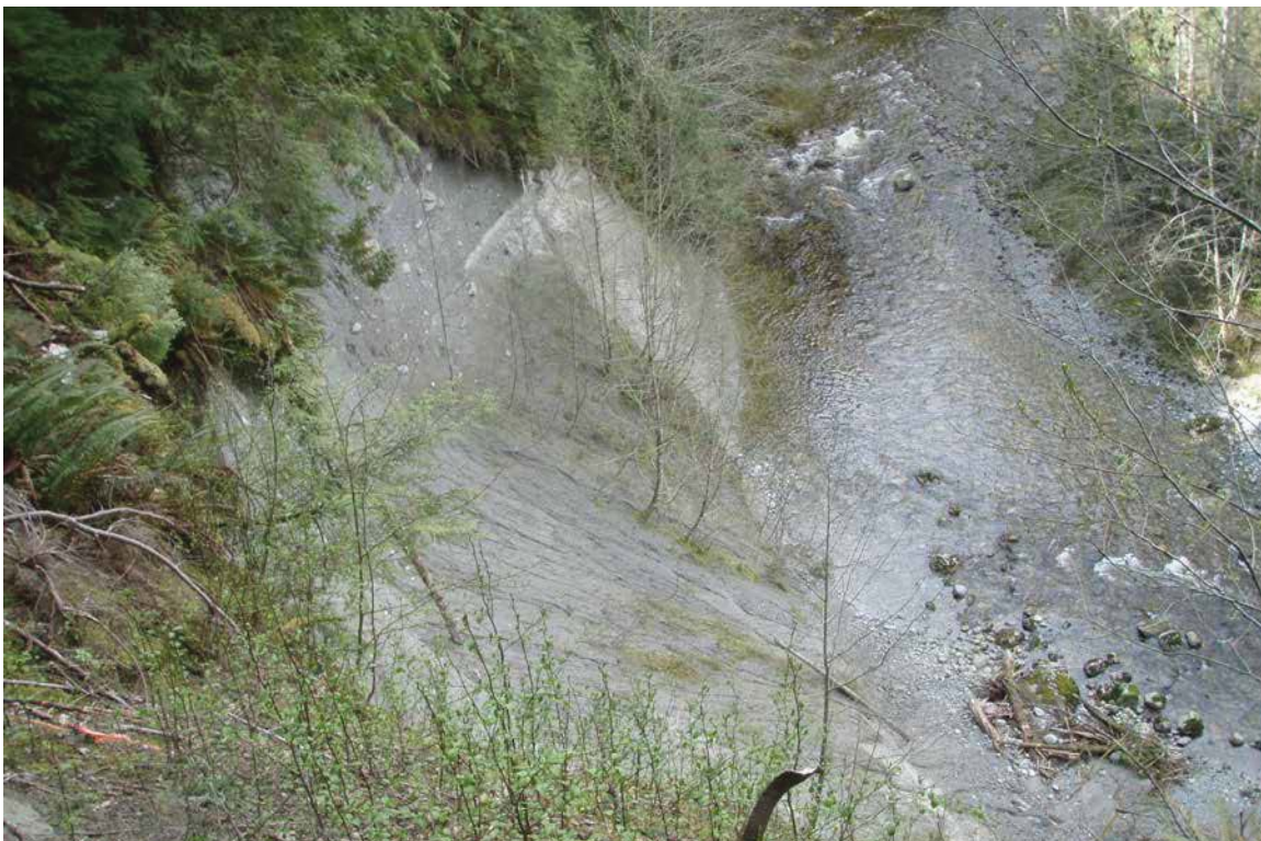
Photo 4 Eroding Bank on Bend Upstream of Chapman Creek Fan
