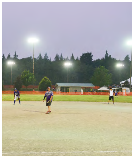
Lower Kinnikinnick field lighting, West Porpoise Bay
