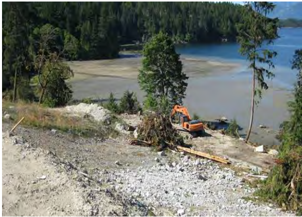
✘ Clearing adjacent to the shoreline should be avoided and upland vegetation retained.
